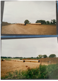
Gas pipes being laid through Great Canfield – crossing Green Street near Deal Tree Farm, August 2002.
